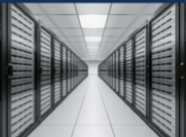
Data Center Cooling
