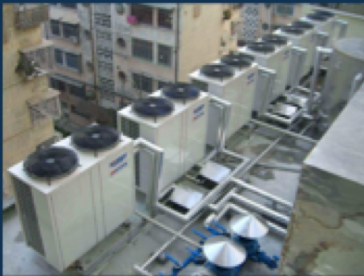
Commercial Building A/C
